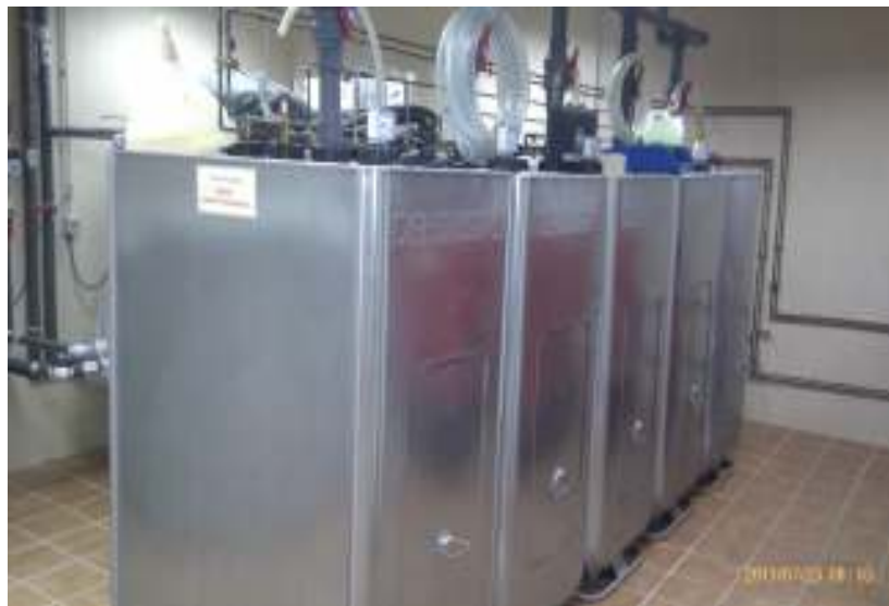
Machine room. Foreground: Double walled oil tanks (Dehoust ®), total capacity up to 5.000 litres. Background right: pipes for boiler & generator fuel supply. Background left: solar heat exchanger for radiant floor (winter season), pipes, valves, temperature probe & circulator.
