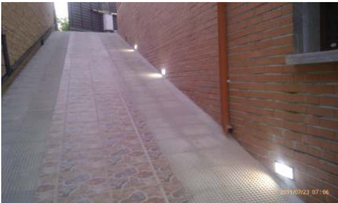
North ramp. Close-up bottom right: night lights automatically lit when swinging motorized door opens for vehicles entrance (foreground up).
