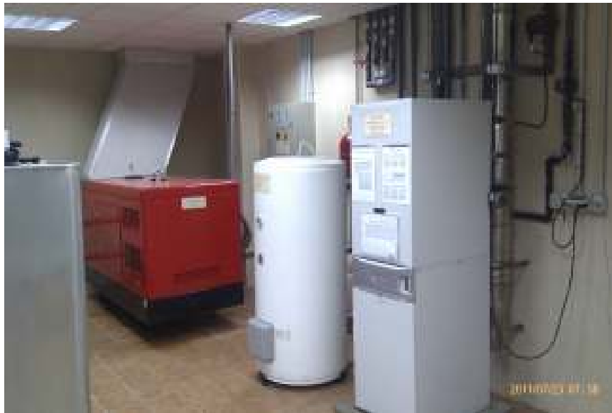
Machine room. Foreground: Boiler & solar heat exchanger for sweet water, fumes chimney, temperature probe, pipings & valves. Behind (not visible), solar panels circulators for pools heating & steam expansions tanks. Background: isolated tree-phase electrical generator (30KVAR), fumes evacuation and automatic control panel.
