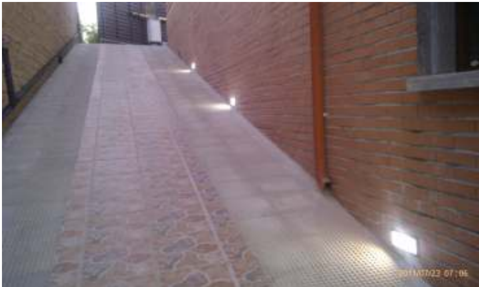
North ramp. Close-up on the lower right: ramp lighting for nighttime vehicle access, with simultaneous ignition to the opening of overhead doors at Mistral Street level. Bottom left: tilting door No. 2 semi-open.
