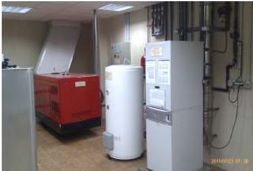
Machine room. Front: boiler and solar exchanger for drinking water, smoke evacuation chimney, temperature probe, pipes and valves. Behind (not visible), solar panel circulator for heating and expansion tanks. Background: isolated three-phase generator (30KVA), smoke evacuation and automatic control panel.
