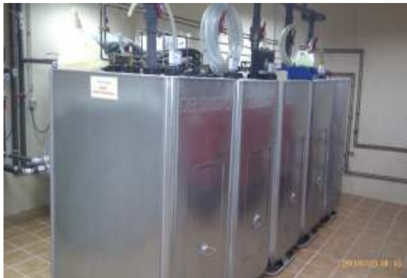
Machine room. Front: double bucket diesel tanks (Dehoust ®), total capacity up to 5,000 liters. Bottom right: diesel feed for the three-phase group and the boiler. Bottom left: solar exchanger for underfloor heating (winter), circuit, valves, temperature probe and circulator.
