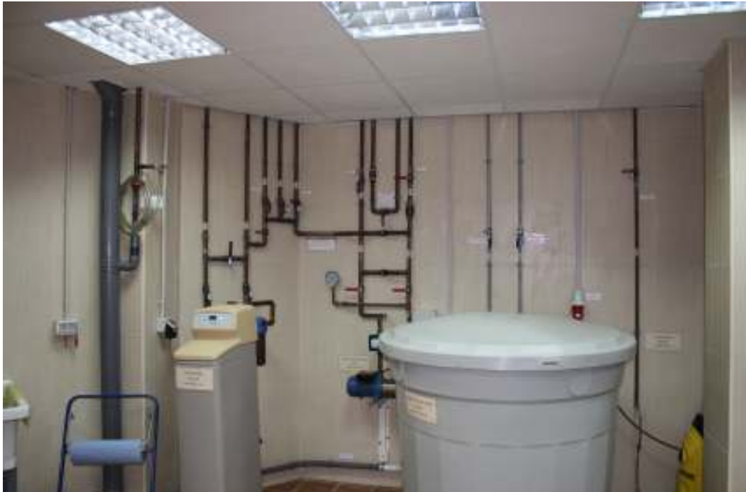
Machine room. Main drinking water supply area, showing storage tank (1 Ton), softener (dry brine), booster pump with pressure stabilizer, pipes and valves for use and distribution of well water.
