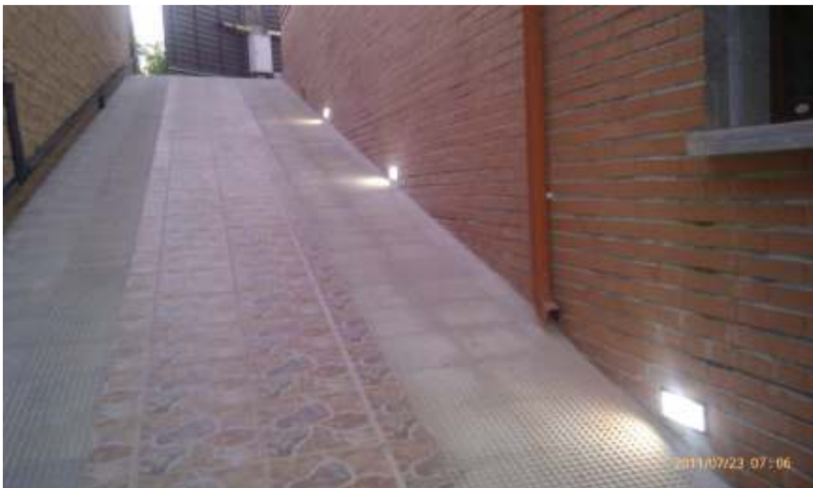
North ramp. Close-up bottom right: night lights automatically lit when swinging motorized door opens for vehicles entrance (foreground up).
