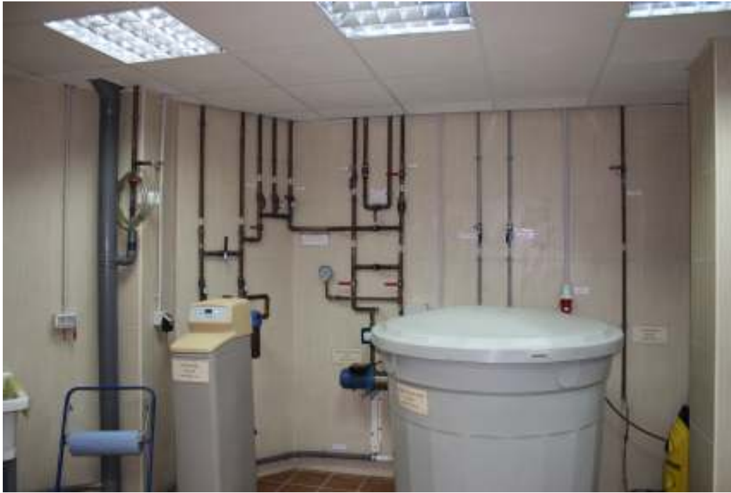
Machine room. Main fresh water supply area, portraying storage tank (1 Ton), water softener (dry brine type), pump & pressure stabilizer, pipings & valves for water well exploitation & distribution.
