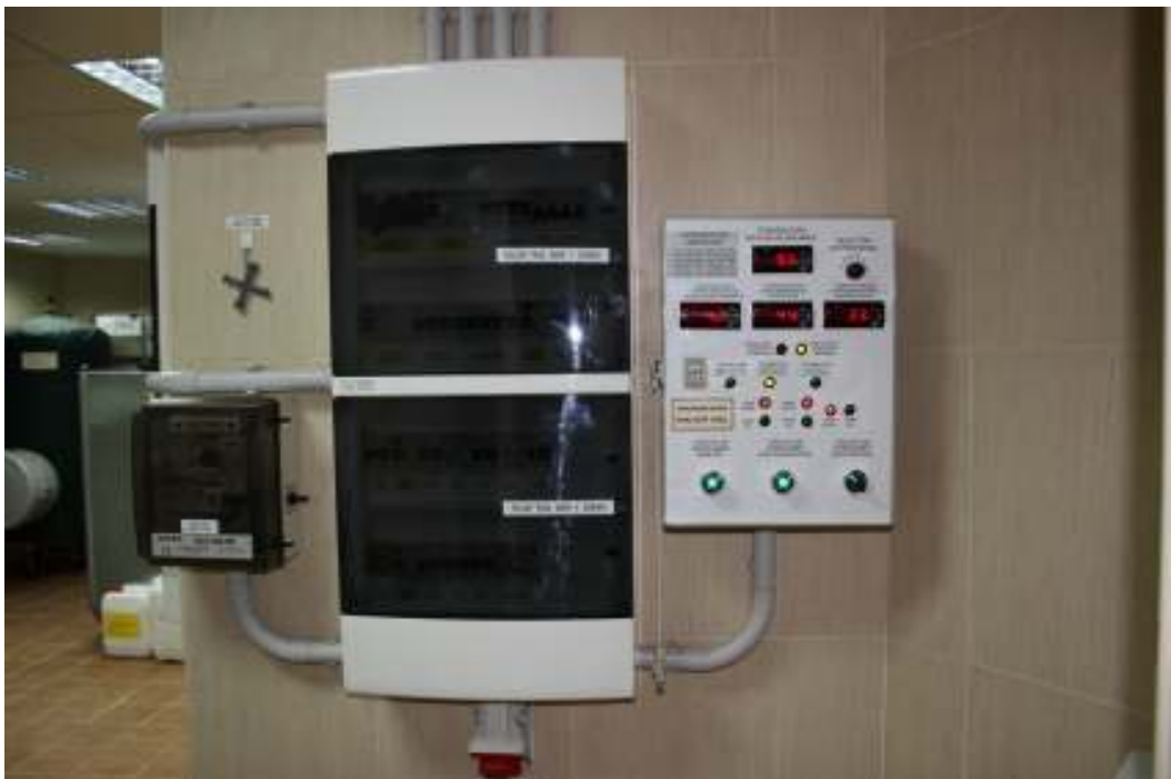
Machine room. Foreground: 3 of 8 control panels. Left to right: water well, main machinery room & solar automaton panel. All breakers and switches are of top quality (Schneider Electric®).
